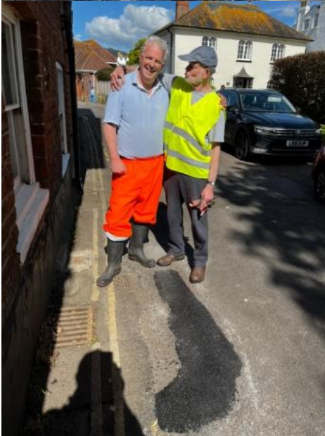
Cheese Lane –(on DCC waiting list for 2 years for this to be done), Ham Car Park entrance, Coburg Road.
