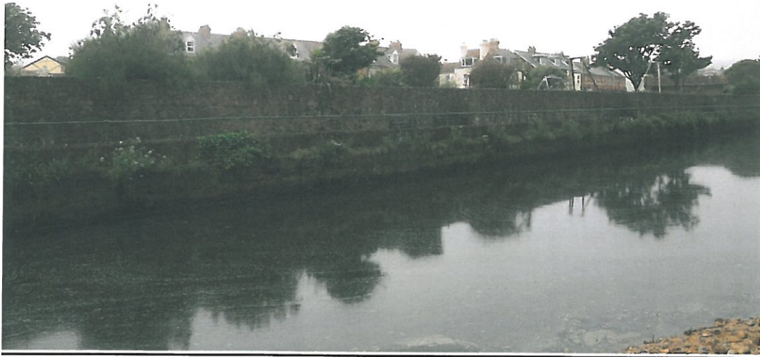
River training walls and EA flood wall behind at the boundary to the Ham
